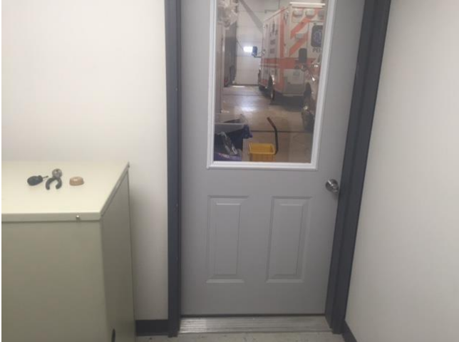
Door between Radio Communication Room & EMS
